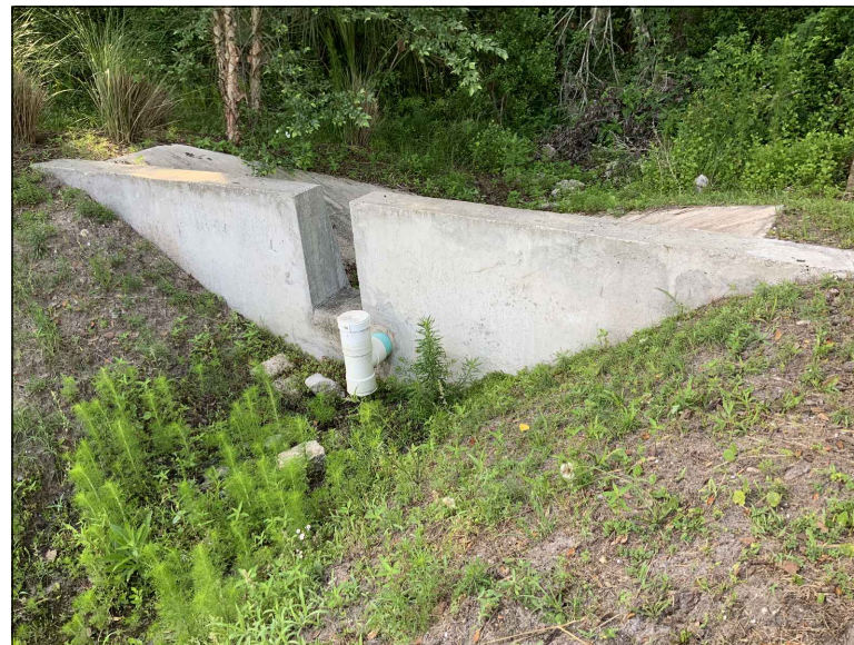
105: VEGETATION GROWING NEAR OUTFALL CONTROL STRUCTURE. IT SHOULD BE REMOVED DOWN TO THE 2'x2' CONCRETE PAD.
