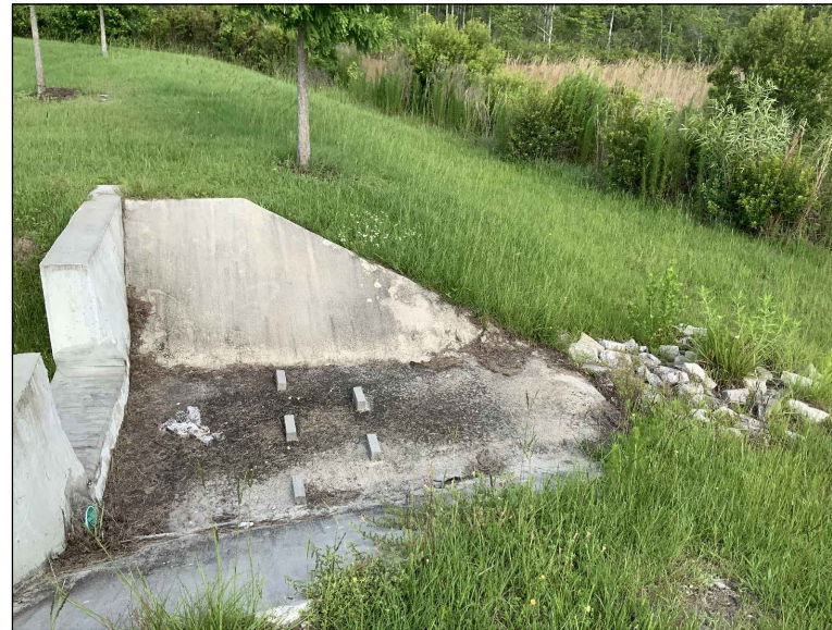
3-5: • OUTFALL CONTROL STRUCTURE HAS MINOR VEGETATION GROWING WITHIN RUBBLE.
