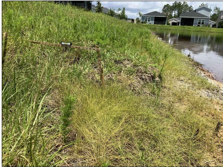
1402: • EXCESSIVE SLOPE NEARING 2:1 ON POND BANK.
