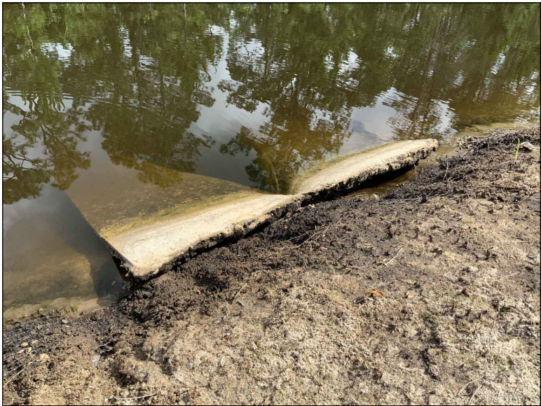
5-5: • CAST-IN PLACE MITERED END SECTION UNDERMINING.
