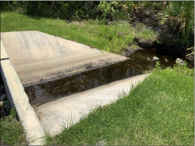
1703: • STANDING WATER IN OUTFALL LOCATION HAS NOWHERE TO FLOW OUT OF SYSTEM.
