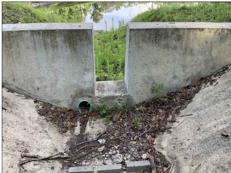
104: DEBRIS BUILDING ON BACKSIDE OF OUTFALL CONTROL STRUCTURE.
