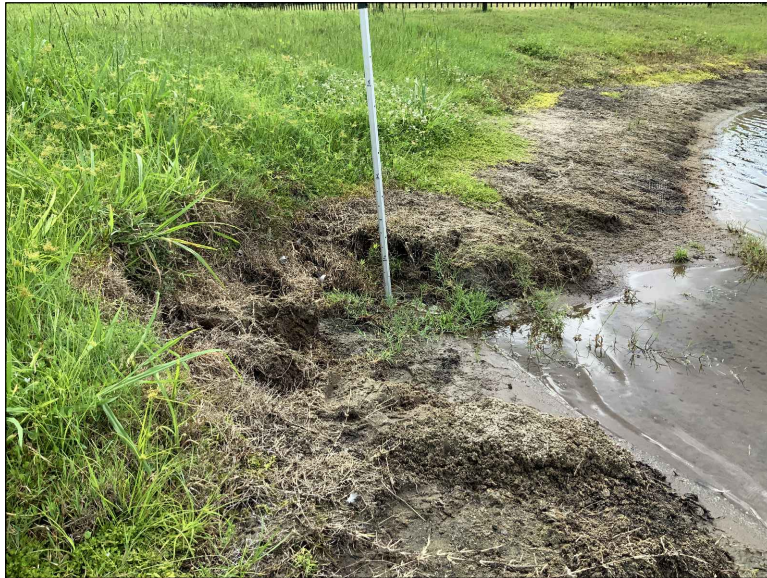
6-2: APPROXIMATE 1.5' DROP-OFF AT NORMAL WATER LEVEL.
