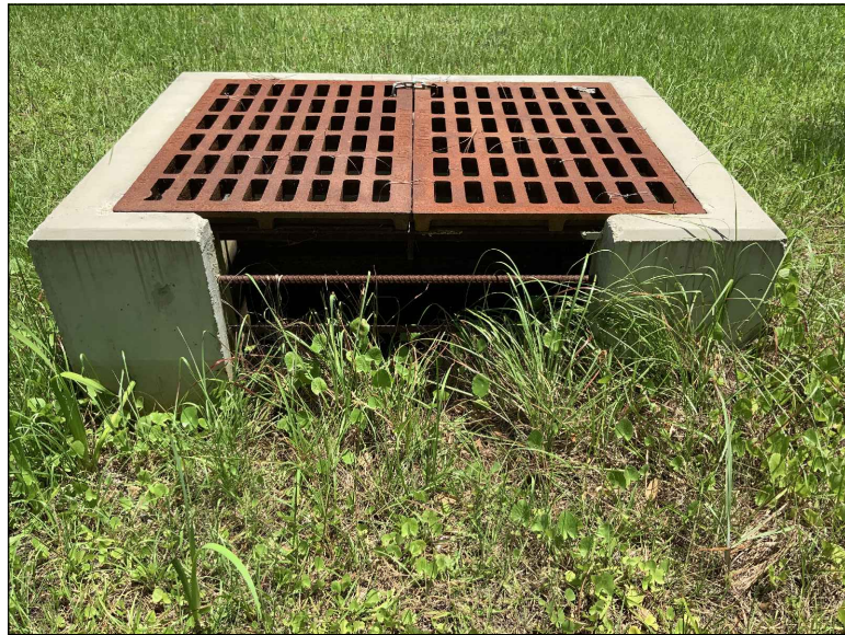
1501: • VEGETATION GROWING IN FRONT OF STRUCTURE'S WEIR.
