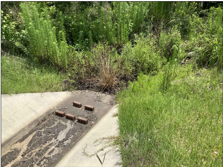
1302: • VEGETATION WITHIN 3'x3' CONCRETE RUBBLE. THERE IS NOT ENOUGH RUBBLE TO COVER 3'x3' AREA.
