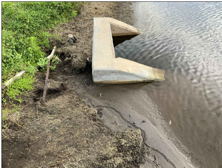
6-5: UNDERMINING BEGINNING ON MITERED END SECTION.
