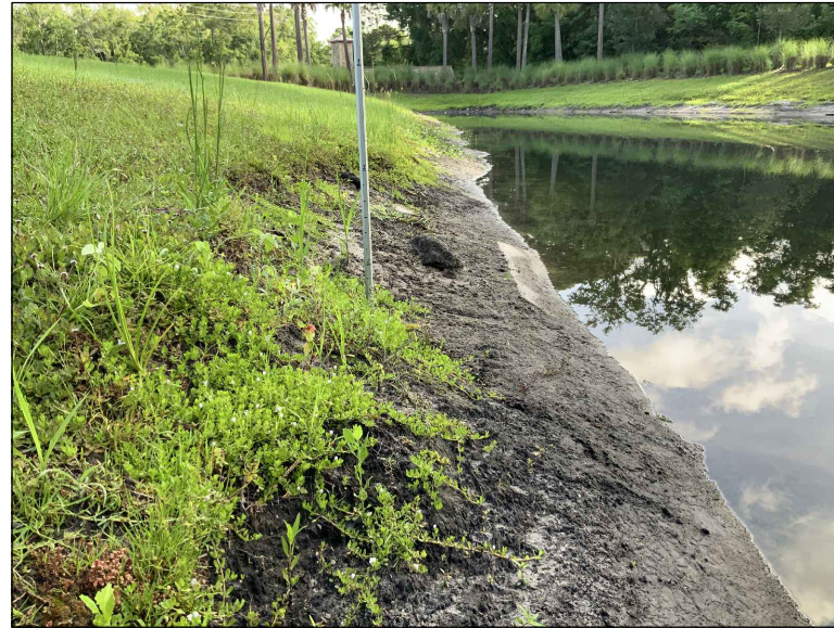
102: APPROXIMATE 1.0' DROP-OFF AT NORMAL WATER LEVEL.
