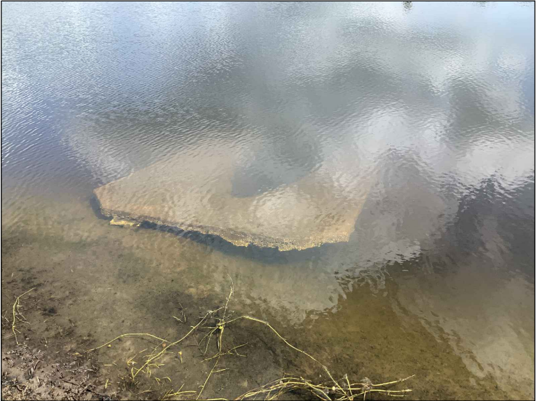
803: • UNDERMINED MITERED END SECTION
