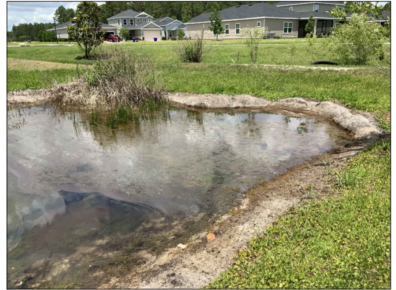
1203: • MINOR VEGETATIVE GROWTH UNDER WATER AND ALONG BANKS OF POND.
