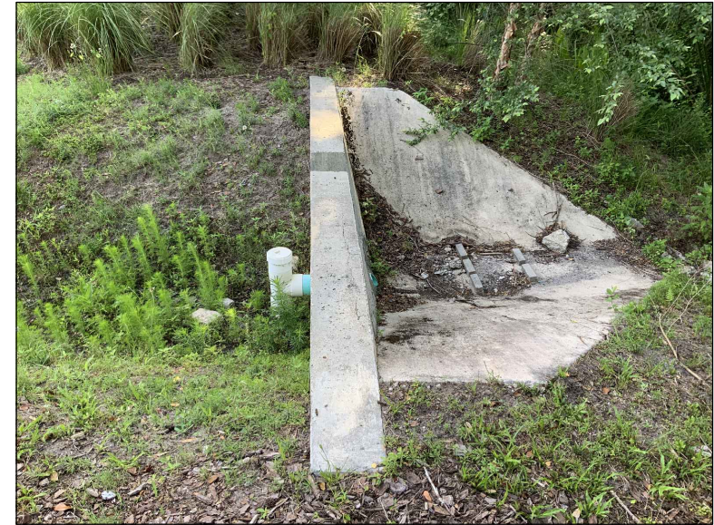
103: OUTFALL CONTROL STRUCTURE HAS VEGETATION AND DEBRIS.
