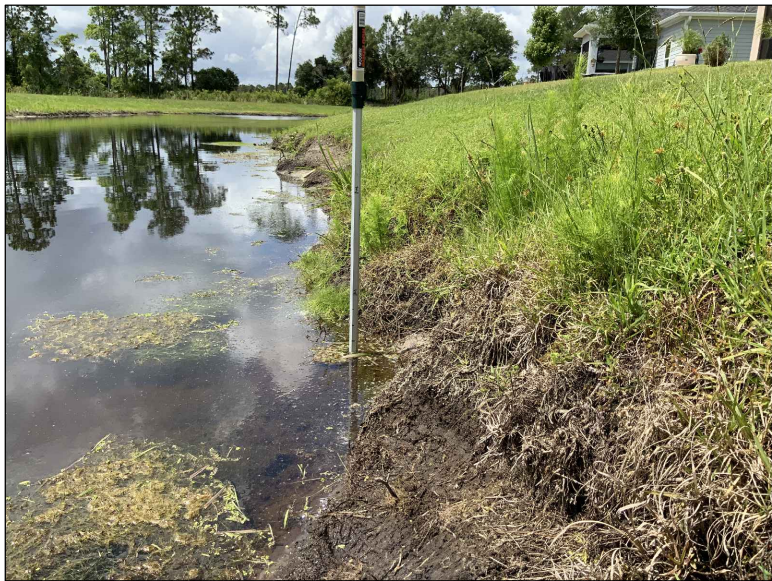
905: 1.5' DROP-OFF AT NORMAL WATER LEVEL.
