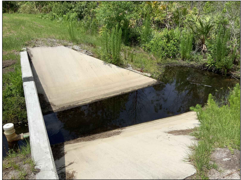
1903: • STANDING WATER IN OUTFALL LOCATION HAS NOWHERE TO FLOW OUT OF SYSTEM.
