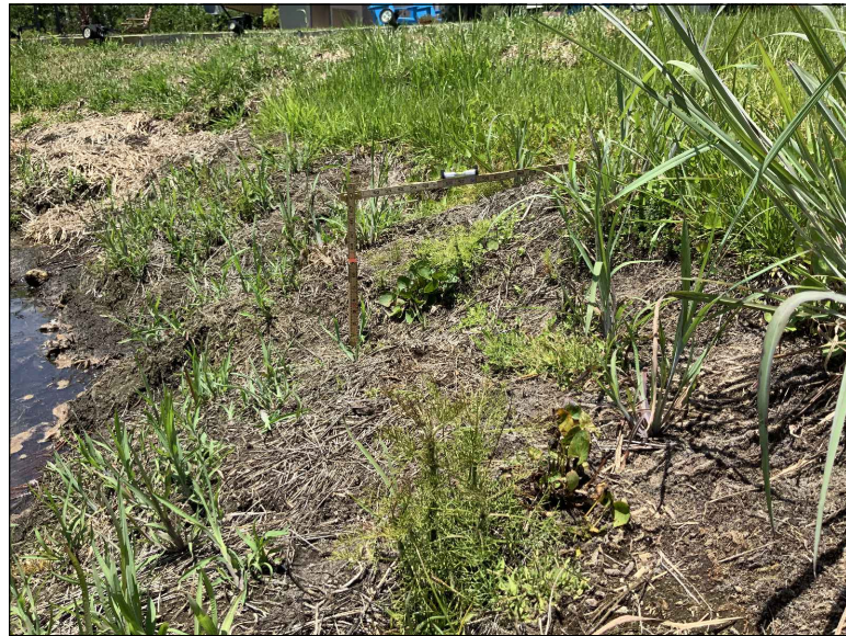
1502: • EXCESSIVE SLOPE ON POND BANK.
