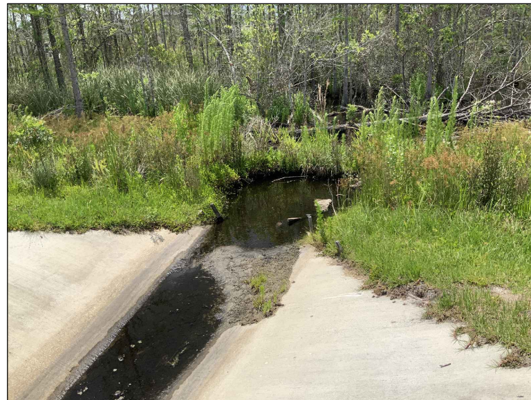
19-5: • OUTFALL LOCATION IS LOWER ELEVATION THAN EXISTING SURROUNDING.
