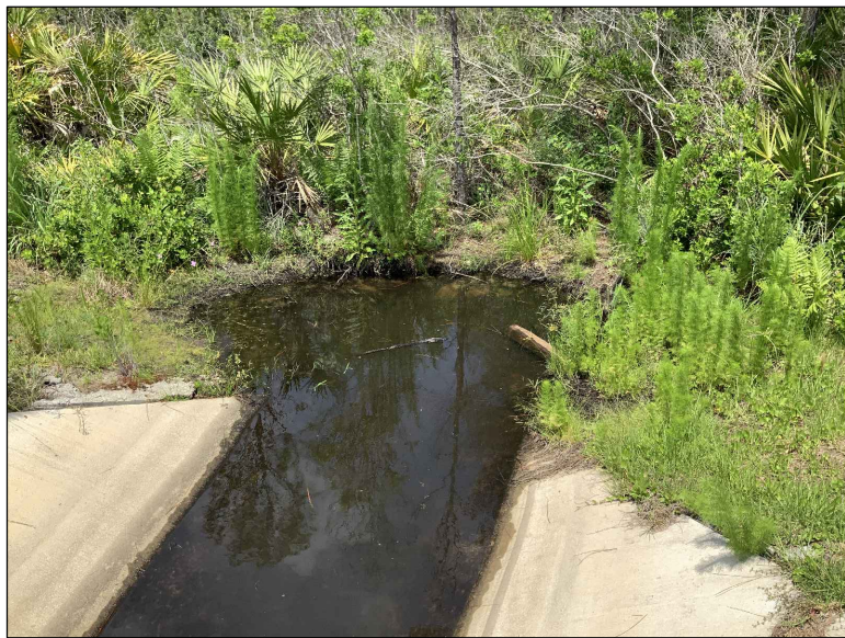
1904: • OUTFALL LOCATION IS LOWER ELEVATION THAN EXISTING SURROUNDING.
