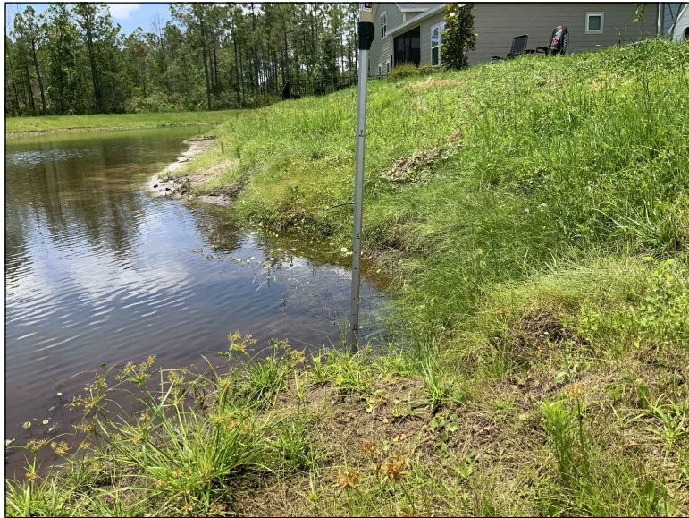
1401: • EXCESSIVE SLOPE AND DROP-OFF AT POND BANK.
