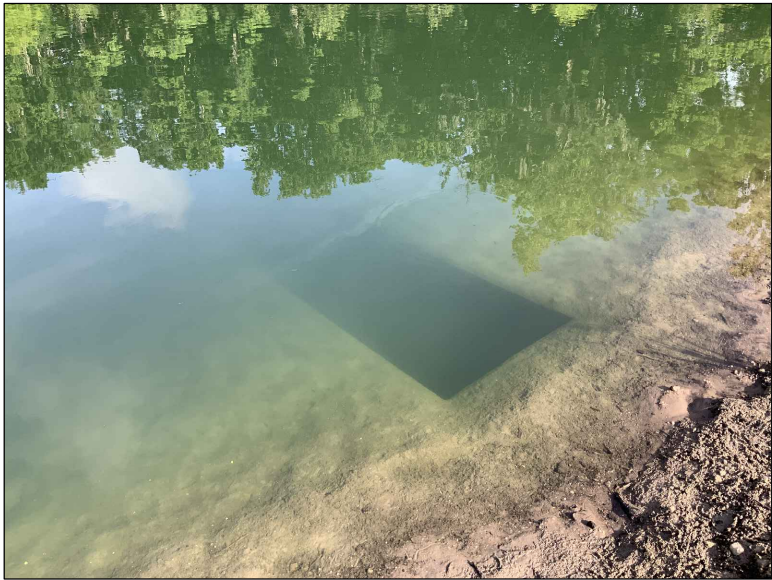
203: MITERED END SECTION CLEAR OF DEBRIS/VEGETATION.
