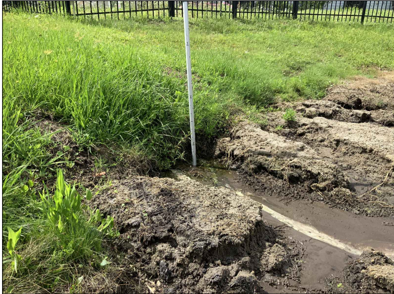
802: • CHANNELING EROSION BETWEEN LOTS
