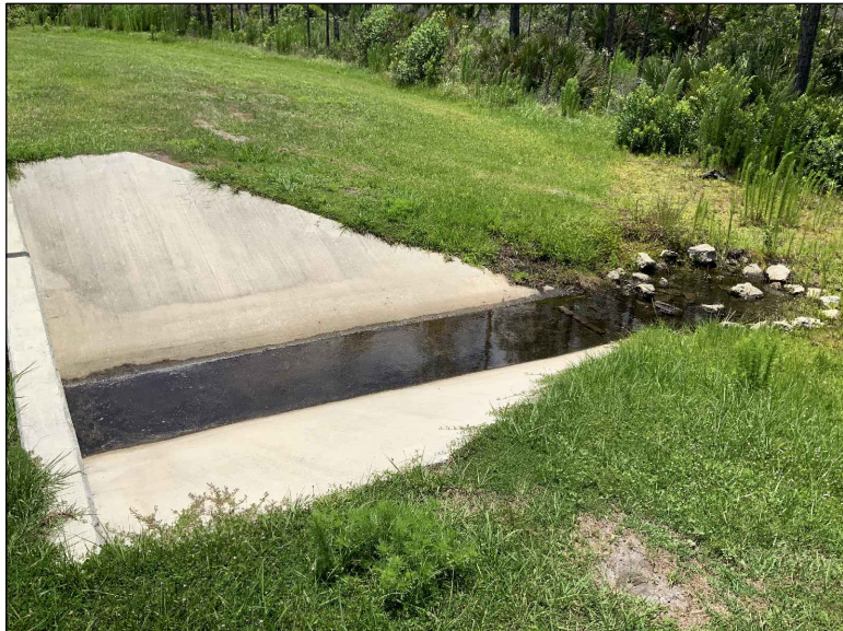
1804: • STANDING WATER IN OUTFALL LOCATION HAS NOWHERE TO FLOW OUT OF SYSTEM.
