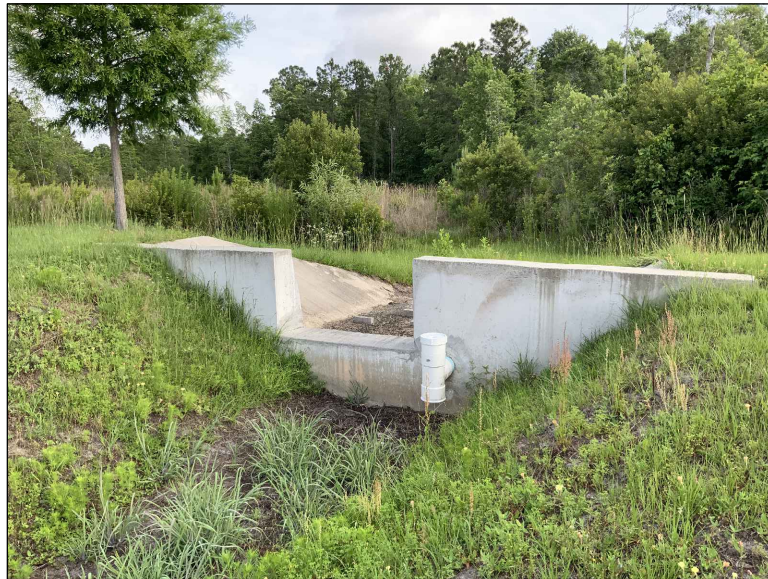
3-4: • MINOR VEGETATION BUILDING IN FRONT OF STRUCTURE.
