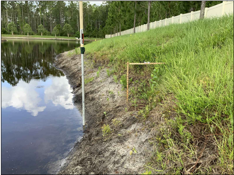
5-2: • EXCESSIVE SLOPE NEARING 1:1 ON BANKS.
