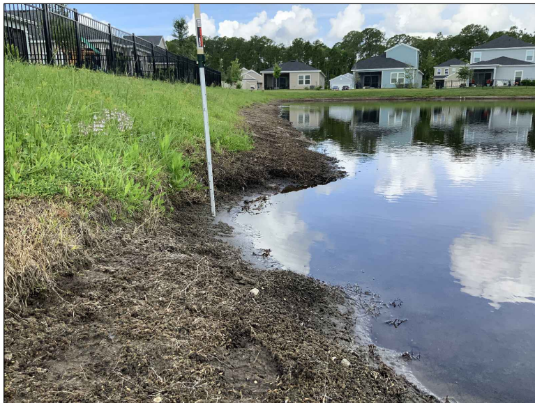
6-4: APPROXIMATE 1.5' DROP-OFF AT NORMAL WATER LEVEL.
