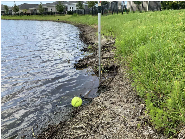
804: • APPROXIMATE 1.5' DROP-OFF AT NORMAL WATER LEVEL
