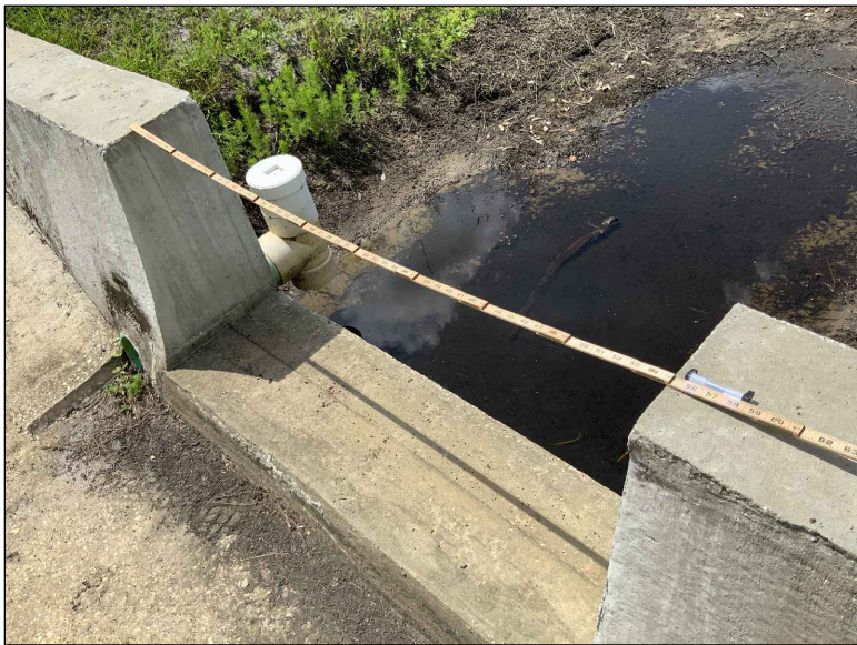
904: OUTFALL CONTROL STRUCTURE WEIR WIDTH MEASURED AT 4.5'. WEIR WAS DESIGNED AND PERMITTED AT 5.5' WEIR WIDTH.
