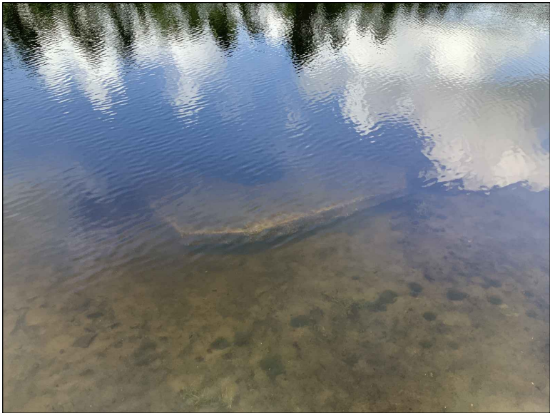
404: • UNDERMINED MITERED END SECTION.
