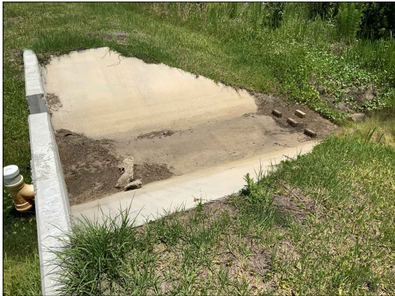
1404: • BRICK ENERGY DISSIPATER MISSING.
