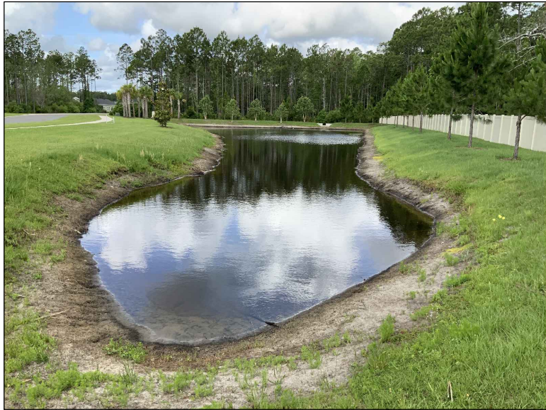
5-1: • EXCESSIVE SLOPES ON BANKS.
