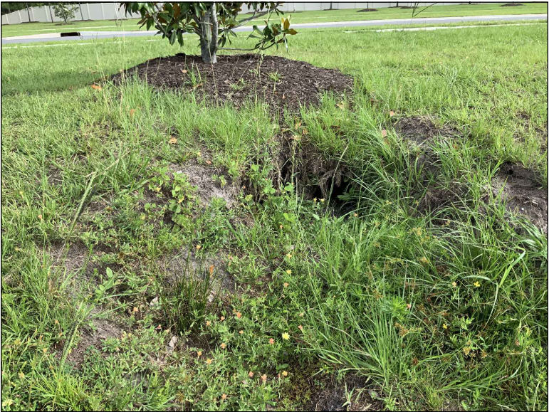
403: • CHANNELING BEGINNING FROM TREE TO POND - POSSIBLE IRRIGATION LEAK LOCATION.
