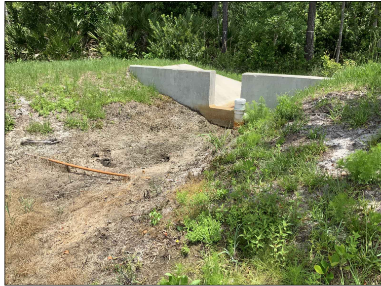
1202: • IRRIGATION LINE CROSSING OUTFALL CONTROL STRUCTURE FLOW PATH.
