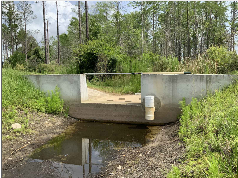
903: OUTFALL CONTROL STRUCTURE WEIR WIDTH MEASURED AT 4.5'. WEIR WAS DESIGNED AND PERMITTED AT 5.5' WEIR WIDTH.
