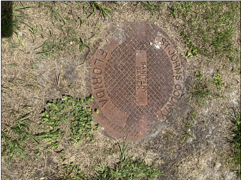
1802: • STORM MANHOLE INSTALLED AS SANITARY SEWER MANHOLE.
