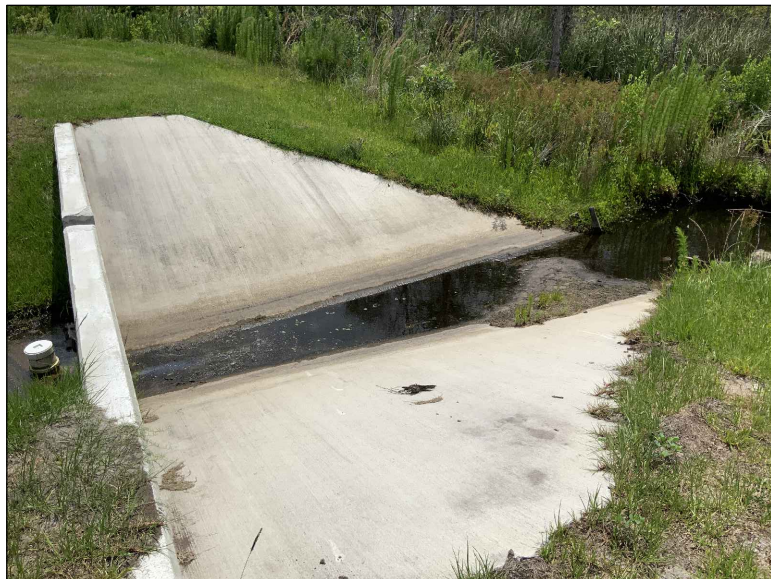
19-4: • STANDING WATER IN OUTFALL LOCATION HAS NOWHERE TO FLOW OUT OF SYSTEM.
