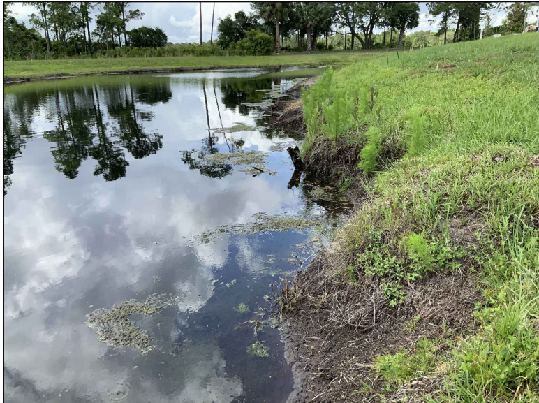
902: 1.5' DROP-OFF AT NORMAL WATER LEVEL.
