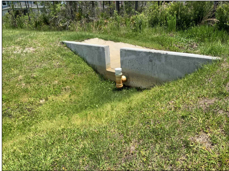
1403: • VEGETATION GROWING WITHIN OUTFALL.
