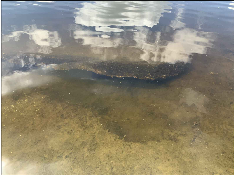
801: • UNDERMINED MITERED END SECTION
