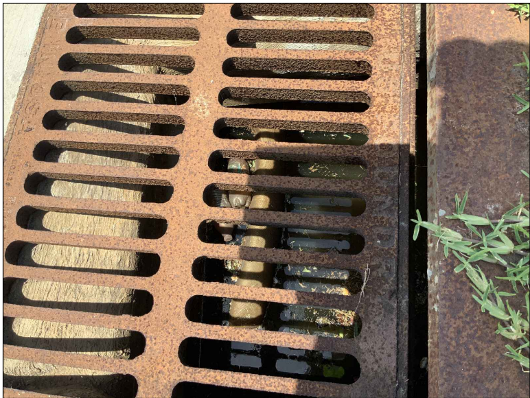
1303: • CURB FILTER FROM CONSTRUCTION WAS WASHED INTO INLET. RECOMMEND REMOVING SO THERE IS NO OBSTRUCTION OF STORMWATER.
