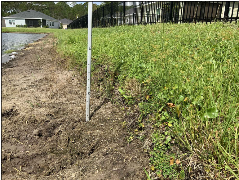
805: • APPROXIMATE 1.0' DROP-OFF AT NORMAL WATER LEVEL
