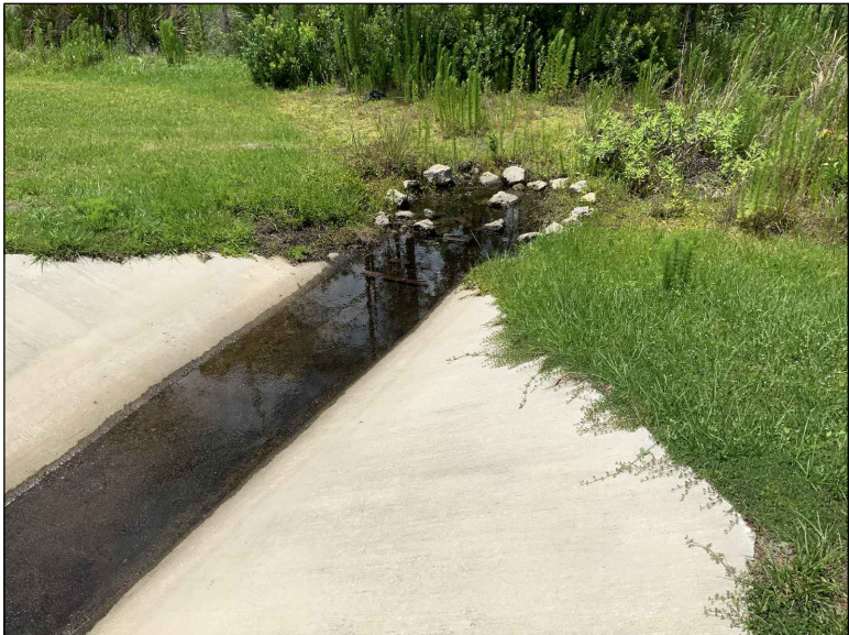
1805: • OUTFALL LOCATION IS LOWER ELEVATION THAN EXISTING SURROUNDING.
