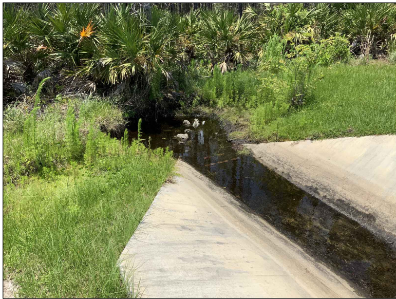
1704: • OUTFALL LOCATION IS LOWER ELEVATION THAN EXISTING SURROUNDING.
