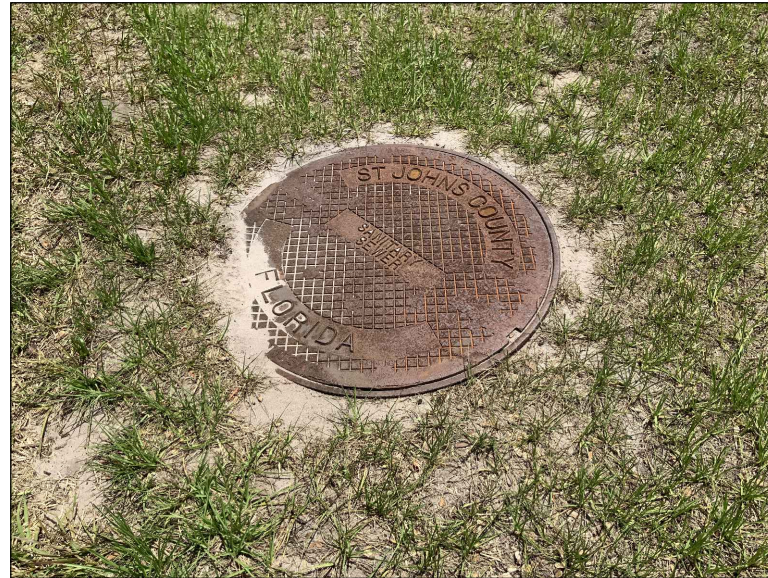
19-2: • STORM MANHOLE INSTALLED AS SANITARY SEWER MANHOLE.
